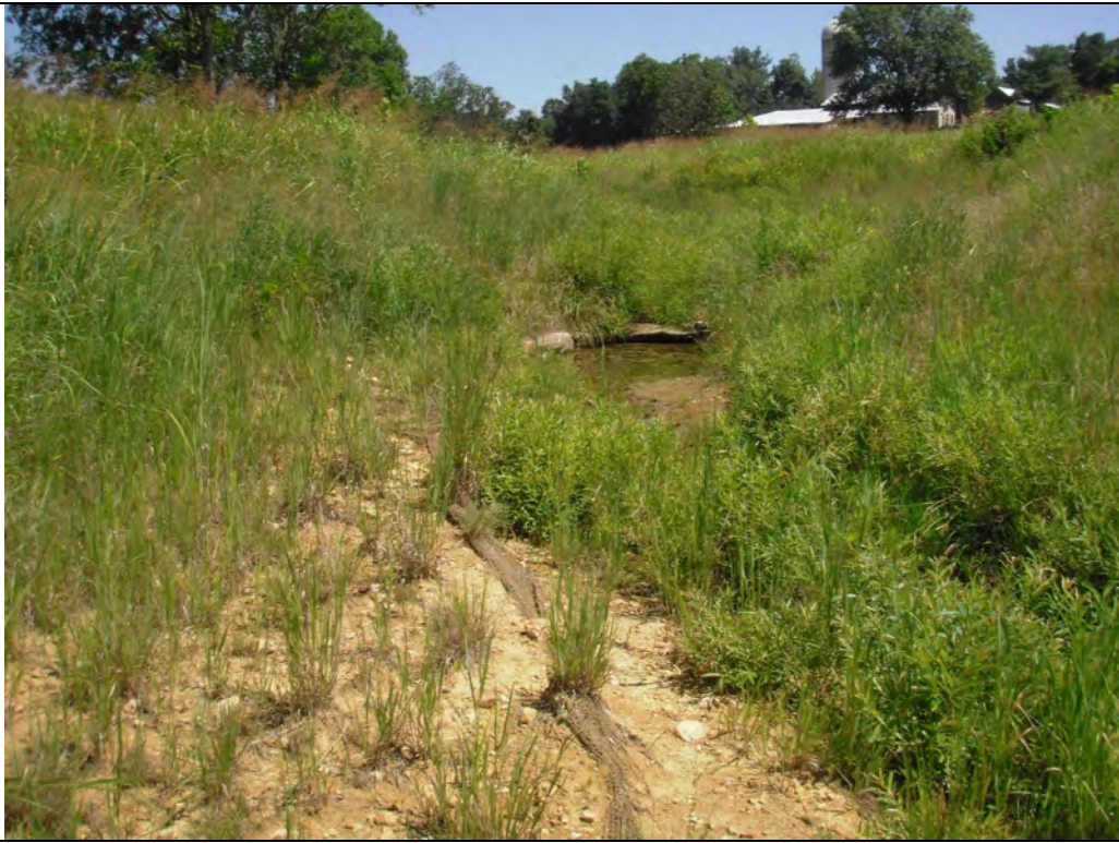
SP5: Bank scour on UTJC1 Taken On: 2010
