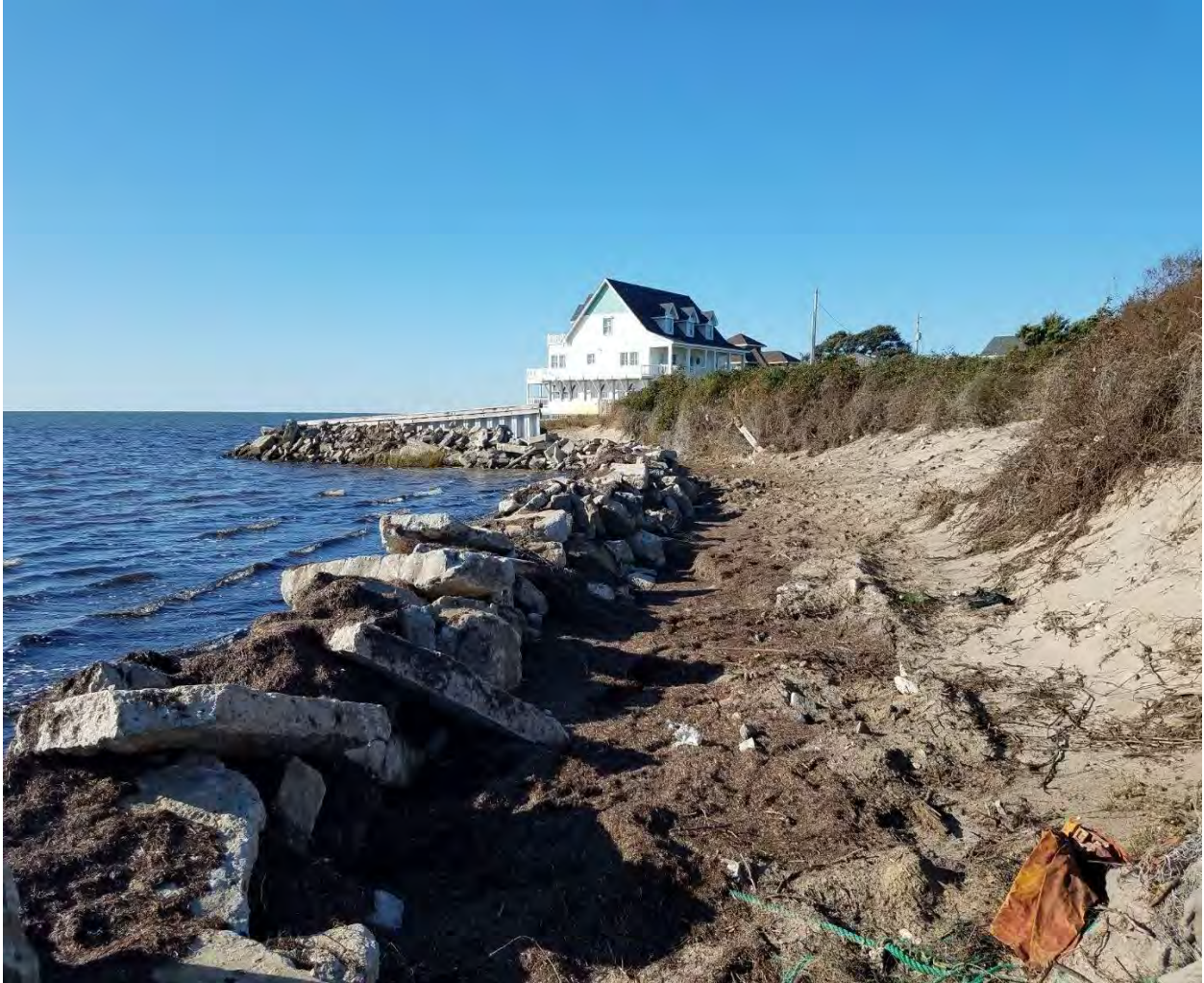
RipRap looking north to the Williams Parcel (now Cahoon) showing the wrack line well beyond the riprap placement.
