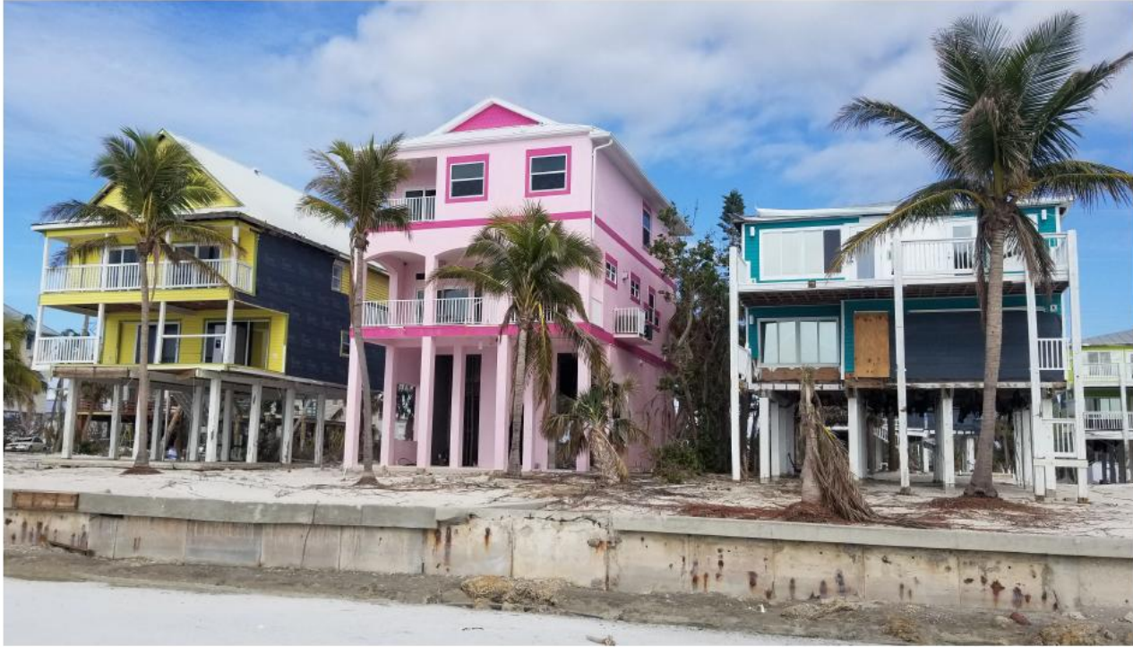
Figure 1: Three neighboring buildings with varying degrees of elevation and damage on Fort Myers Beach, Florida, after Hurricane Ian. The right-most building has the lowest elevation of the three and the most damage to the lower levels, whereas the middle building has the highest elevation and minimal damage to the lower levels.
