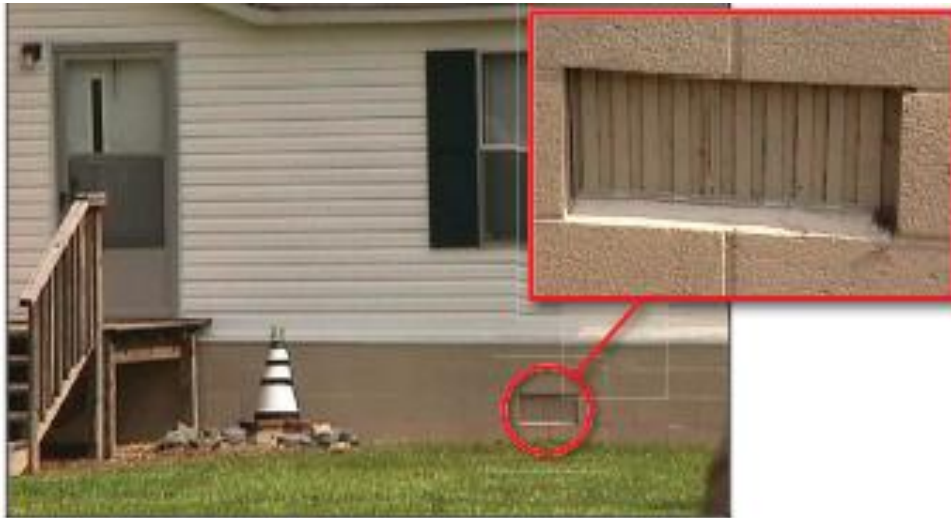
Figure 17: Standard air vent that is unacceptable as a flood opening because it is not disabled in the open position
