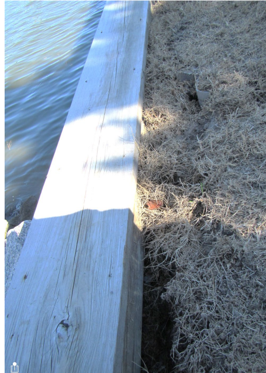
Scour landward of the wall
