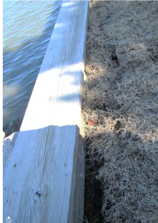
Scour landward of the wall
