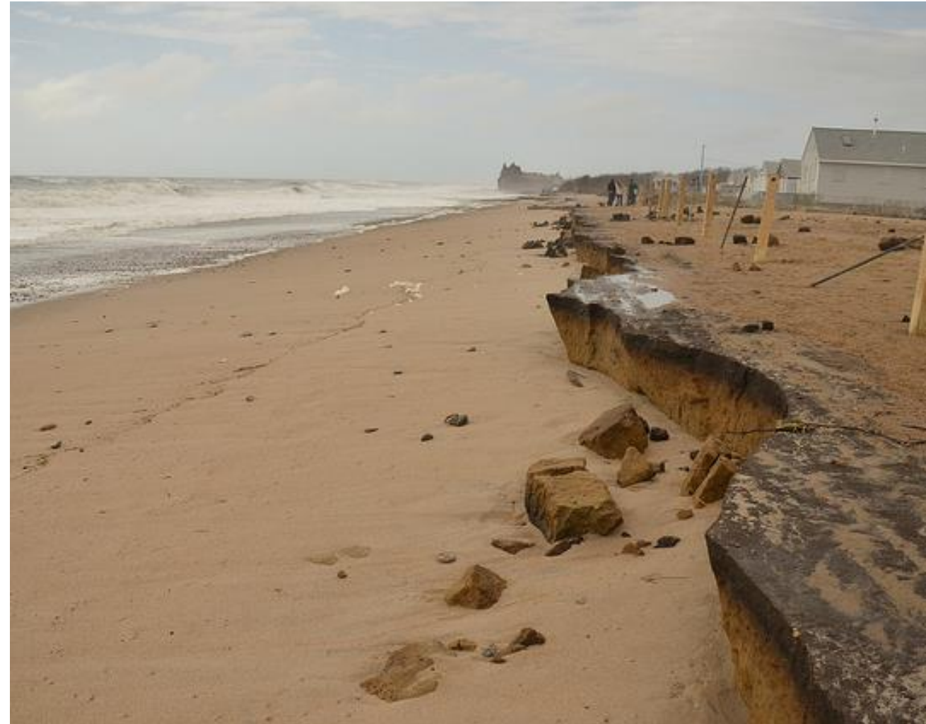
Matunuck post Tropical Storm Sandy (photo credit: CRMC)
