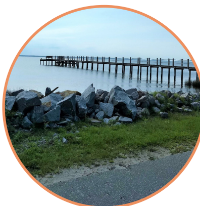
Duck Road is nearly at sea level and protected with rip-rap at a low point.
