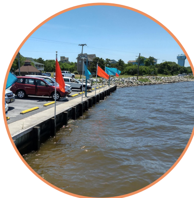
The seawall on this heavily modified shoreline provides scarce habitat and increases localized erosion.
