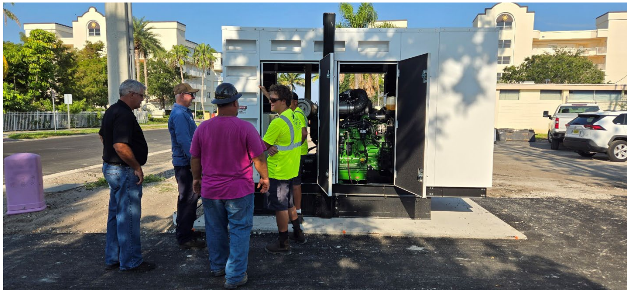
Cape Canaveral Center Street Pump Station
