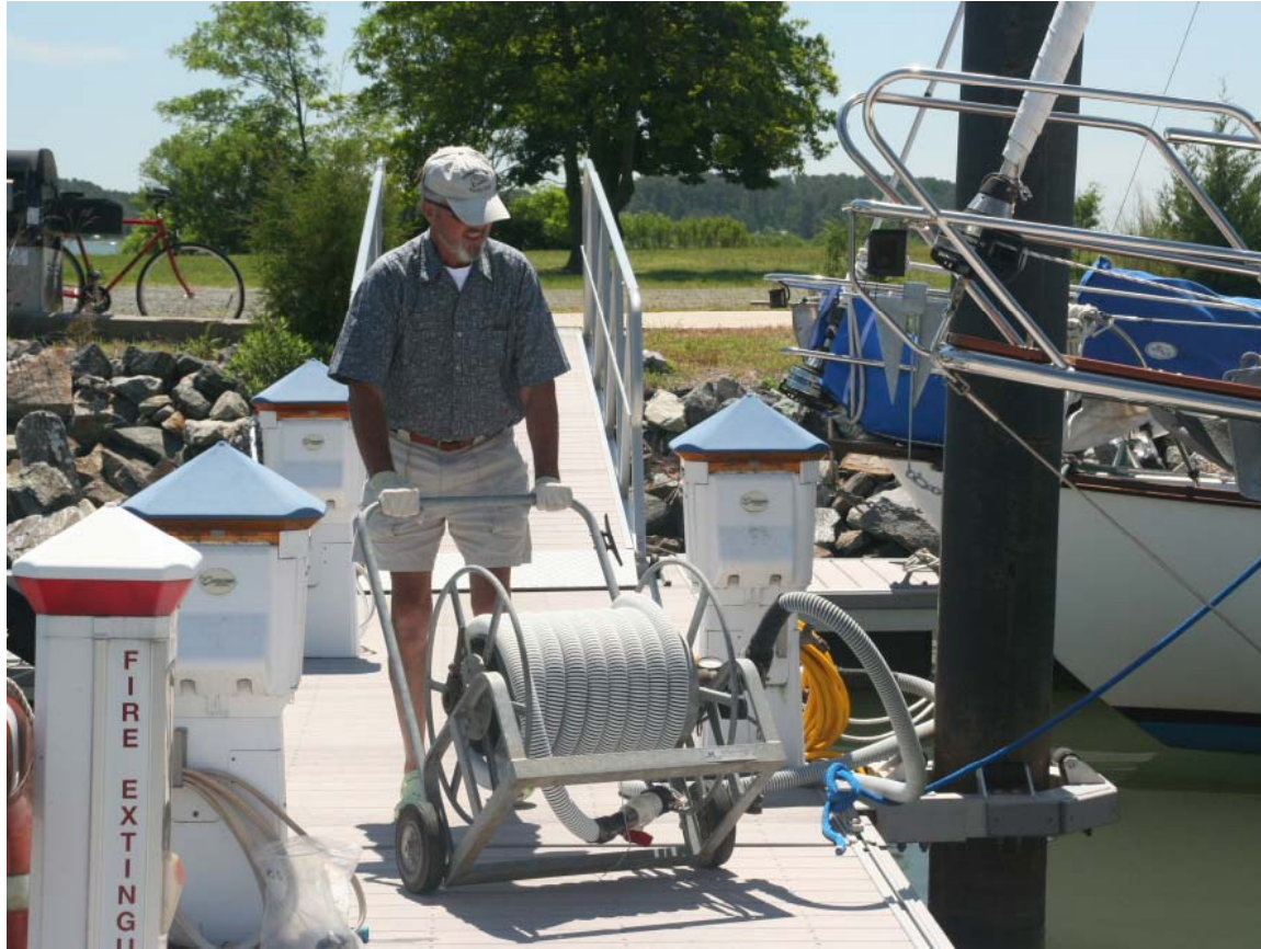
Customer In-Slip Pump Out
