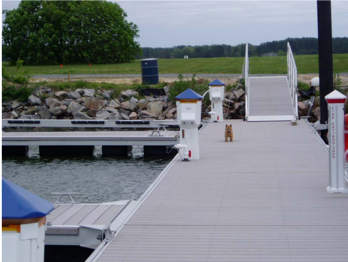
Multi-Point Collection (Suction Hydrants)
