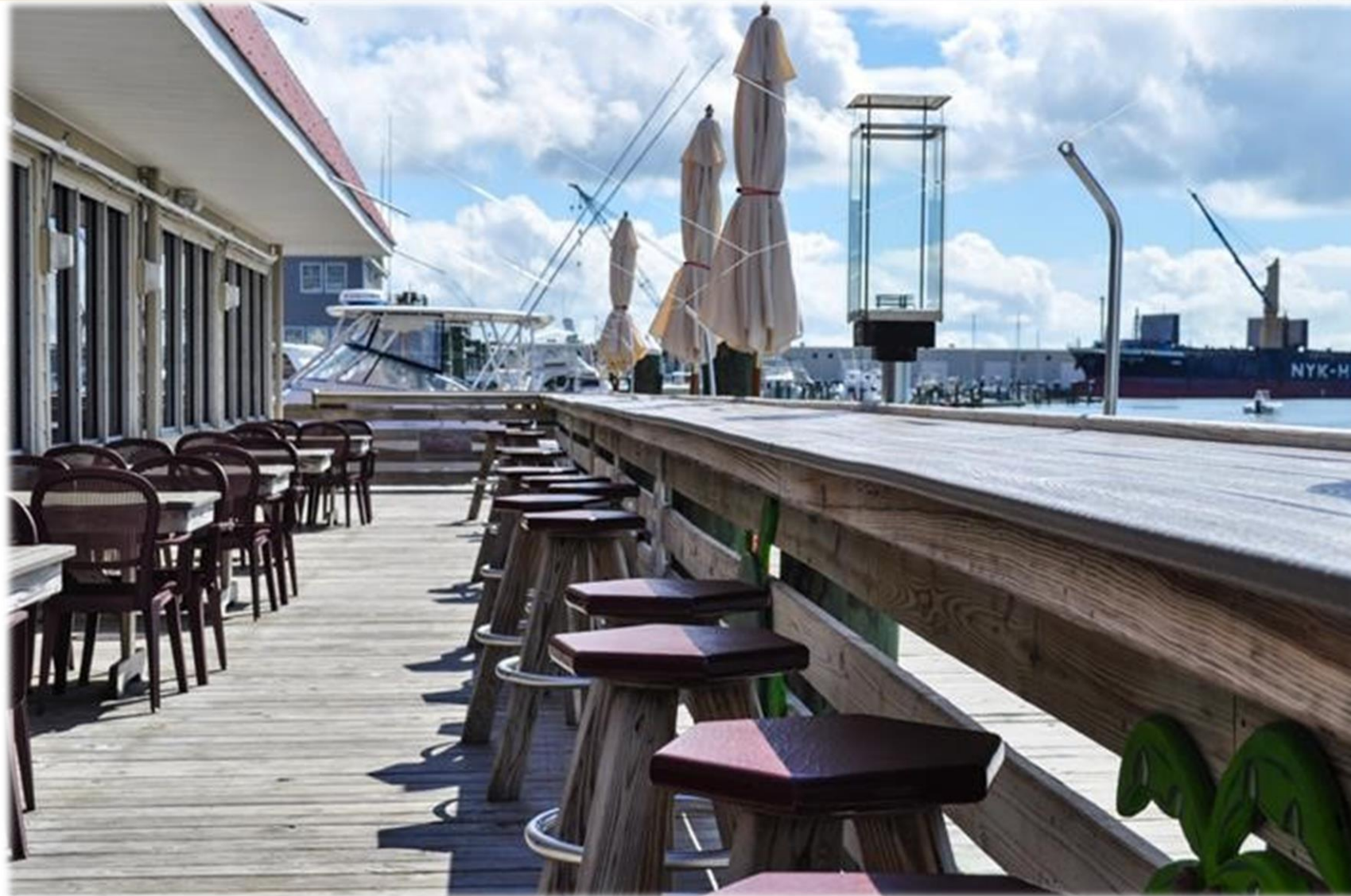
View of existing dock platform area on south side of the Sanitary Restaurant 2015 Photo
