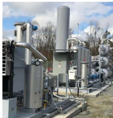
Refinery in Kenansville converts gas from the Optima KV project in Duplin County that pipes in methane gas from hog farms. The gas is used to produce electricity at Duke Energy's Smith Energy Complex in Richmond county.
