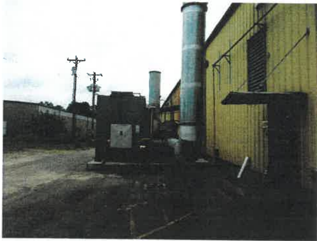
Picture 1: Overall view of the regenerative thermal oxidizer.
