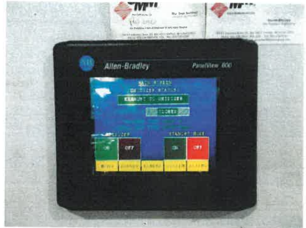
Picture 2: Detail of the new control panel showing the RTO operating at 1514 degrees (F).
