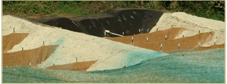
Design Issue: Topography and site conditions sometimes results in plan implementation that was not indicated by the designer. Project personnel coordinate revisions with the Roadside Environmental Field Operations personnel.
