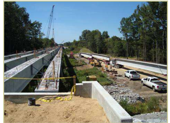
Causeways constructed from timber mats and temporary construction bridges are utilized to protect environmentally sensitive areas during construction.
