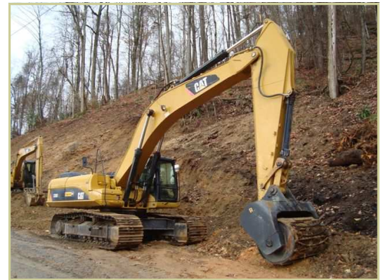
Slope Compactor: The Department field tested a commercially available slope compactor to evaluate its ability to prep slopes for seeding on projects with steep slopes..
