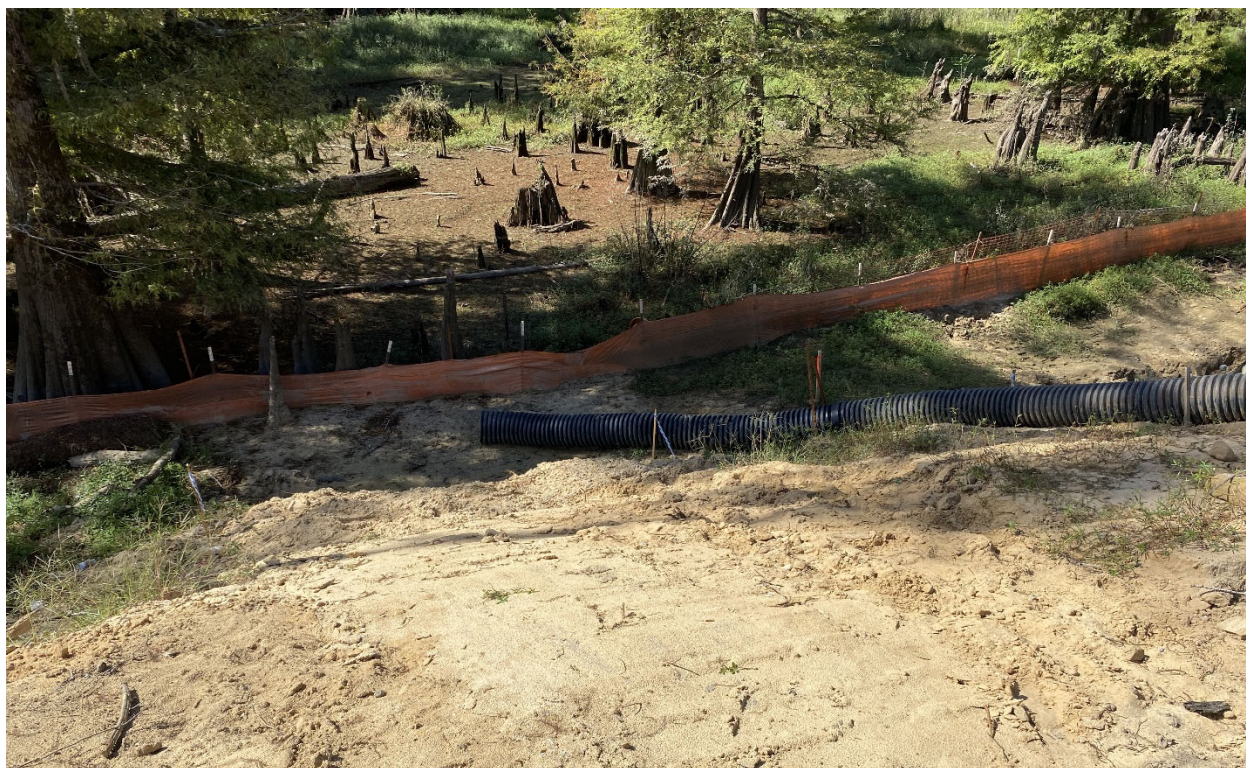
Dissipator pads needed at slope drain outlets.
