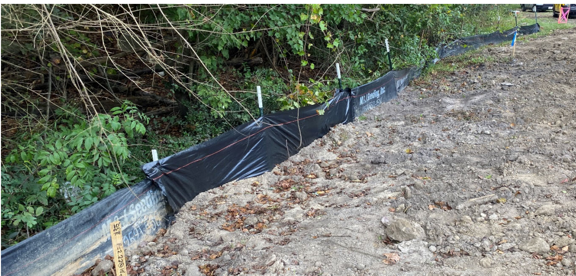
Previous silt fence repairs.
