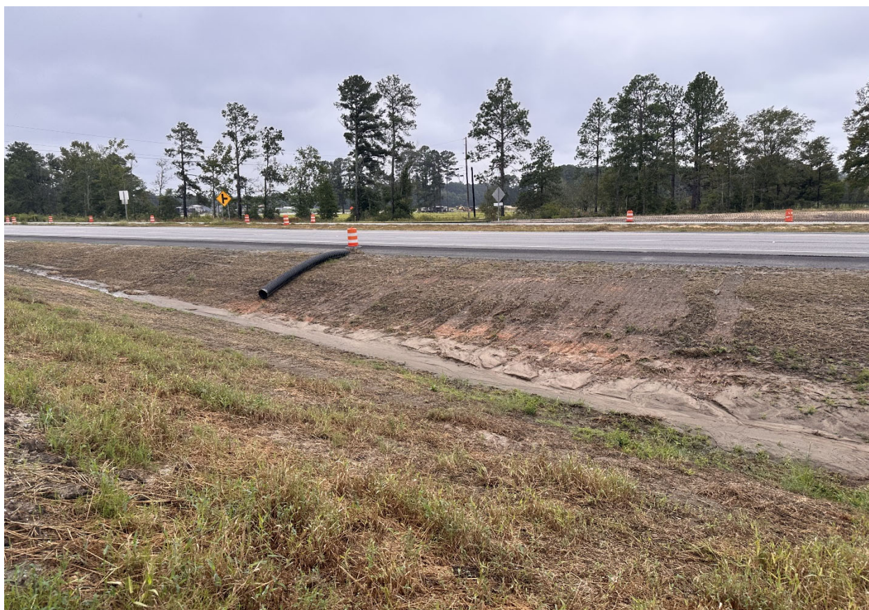
Slope drains need to be extended and dissipator pads installed.
