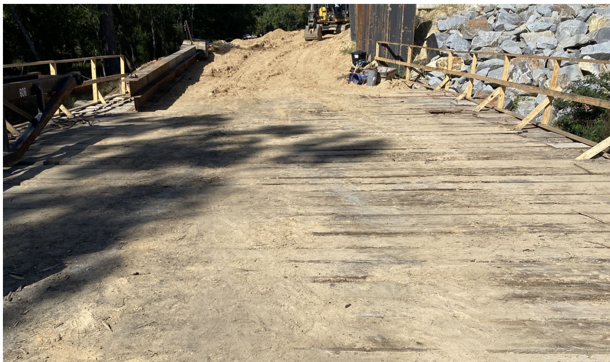
Sediment tracking onto work bridge.
