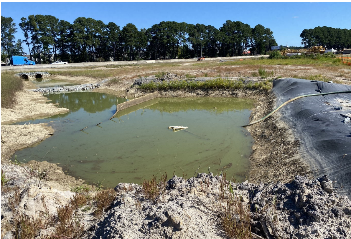
Baffles needing repair.
