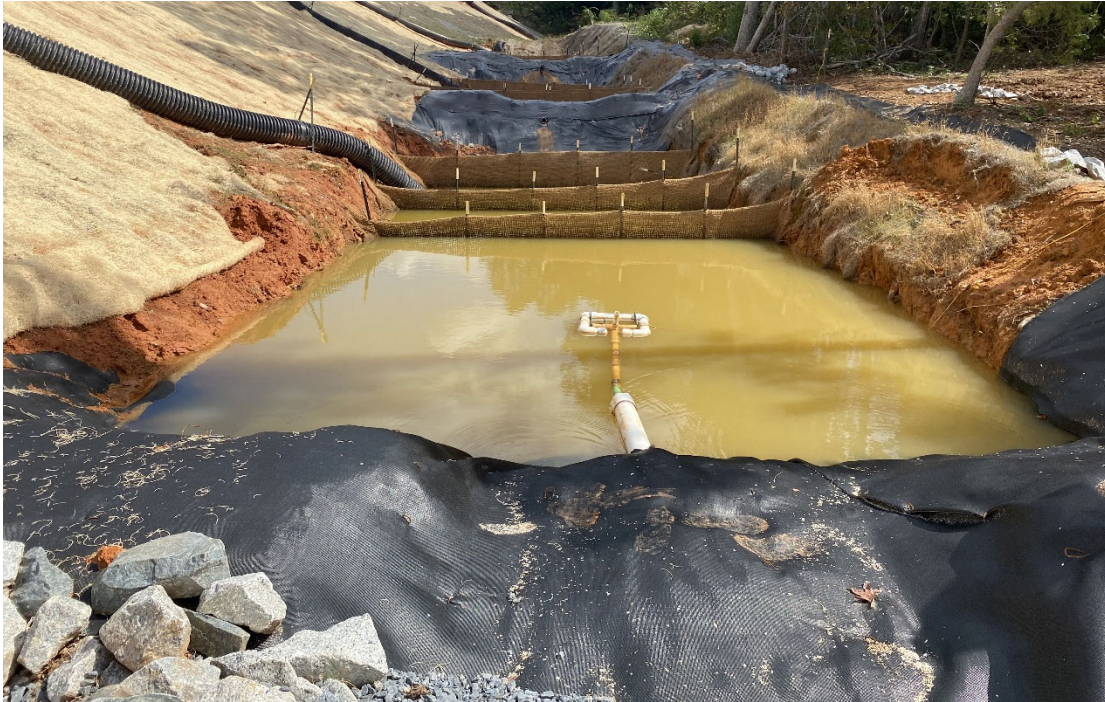
Skimmer basin not fully dewatering and slope drains in wrong bay.
