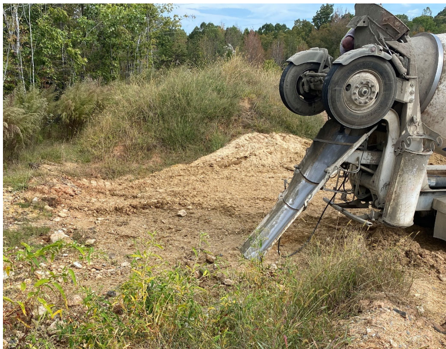
Concrete truck washing out directly on the ground.
