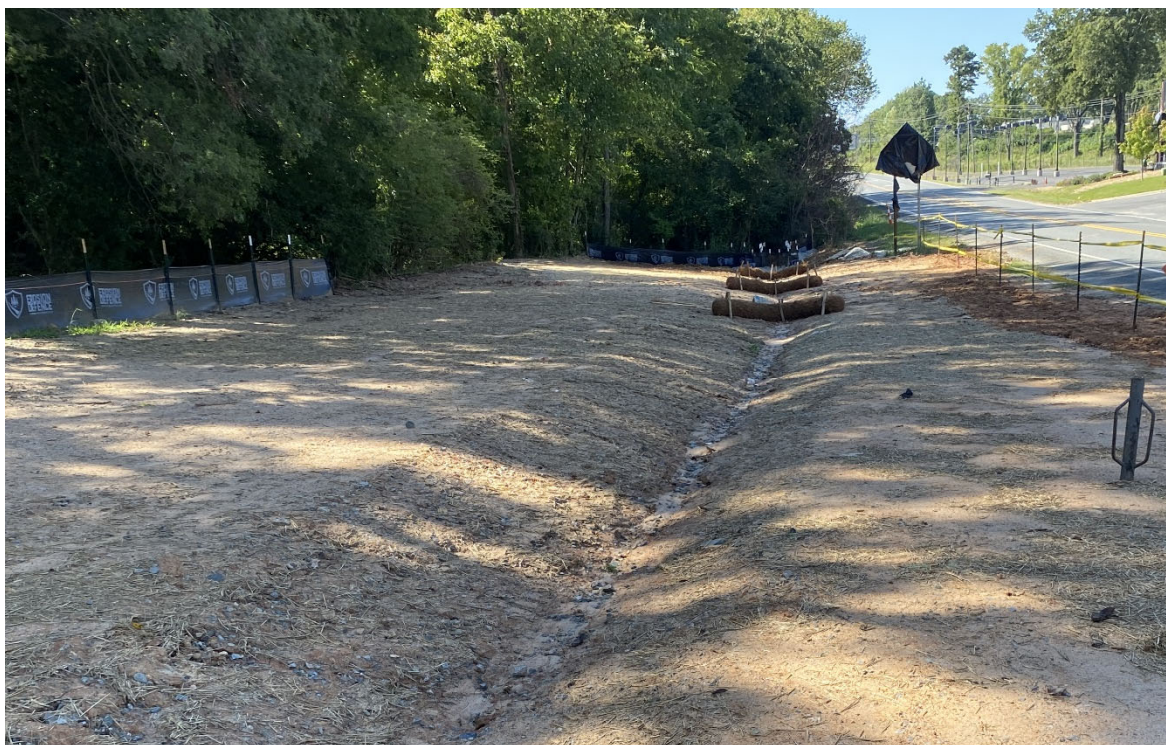
Wattles needed to be properly spaced.
