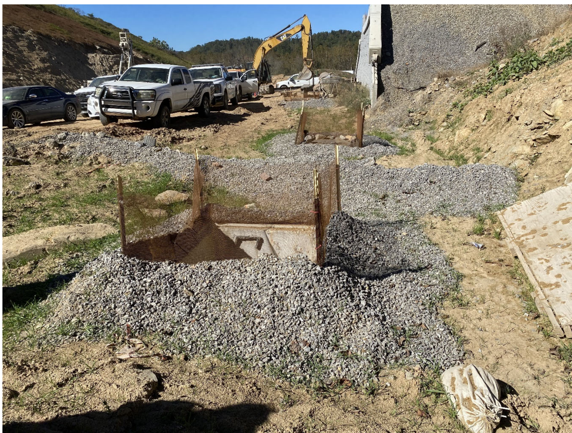
Drop Inlet Protection measures
