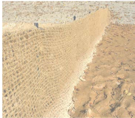
Figure 6.65d Close-up of a porous baffle.
