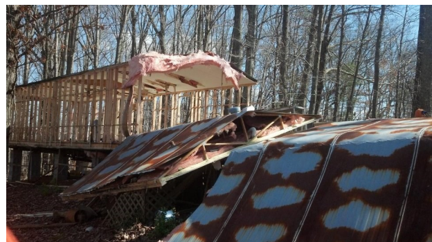
By deconstructing mobile homes by hand, Holt Custom Trailer can recycle up to 90 percent of the home's material.
