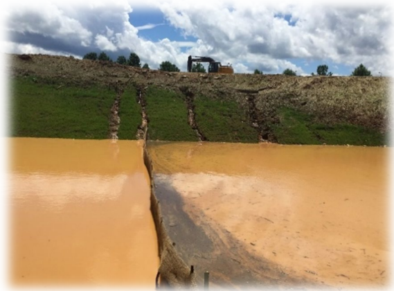
Figure 10 - Rill Erosion on Sediment Basin Slope
