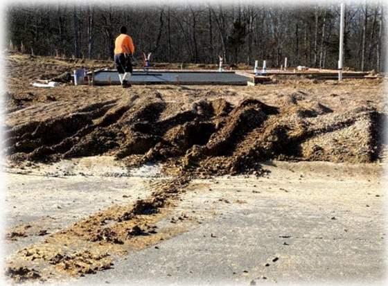
Figure 7 – Poor Construction Entrance
