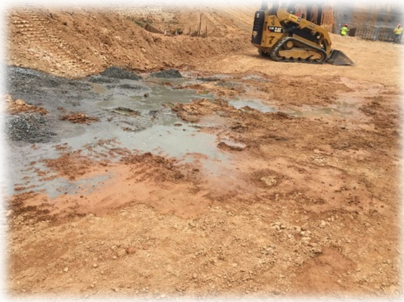
Figure 5 - Unmanaged Concrete Washout
