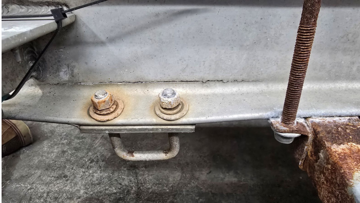
Cracked main frame
