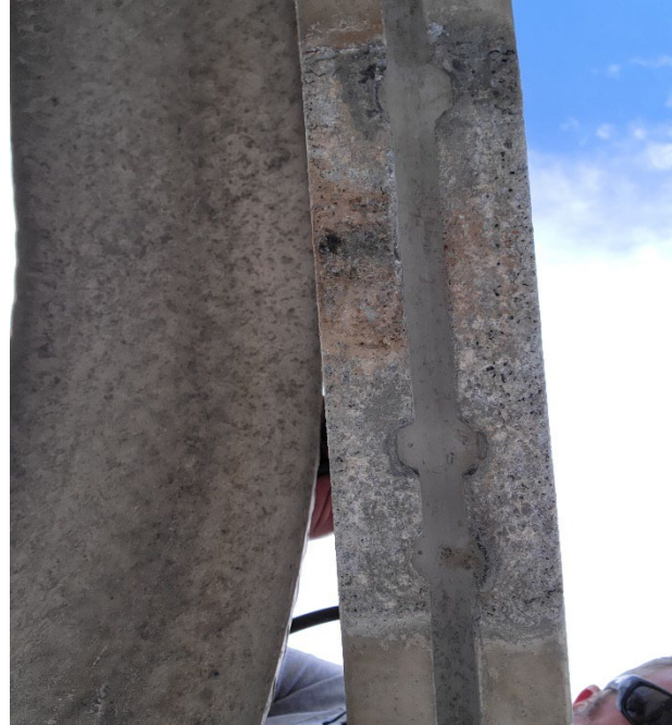
Bolts separating due to cracked frame
