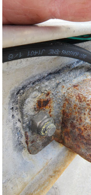
Corrosion inside main frame where cross members meet
