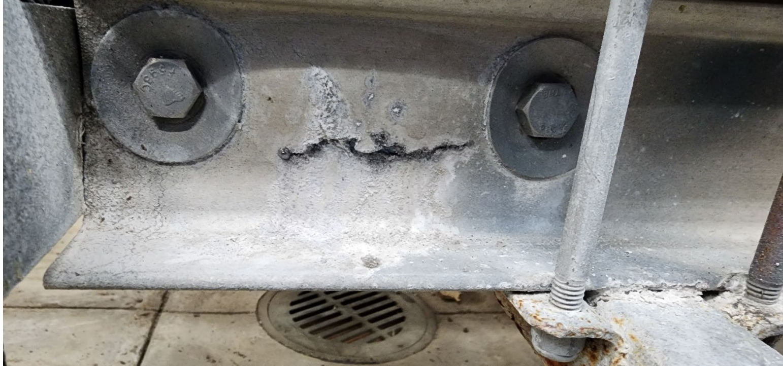
Cracked main frame due to corrosion
