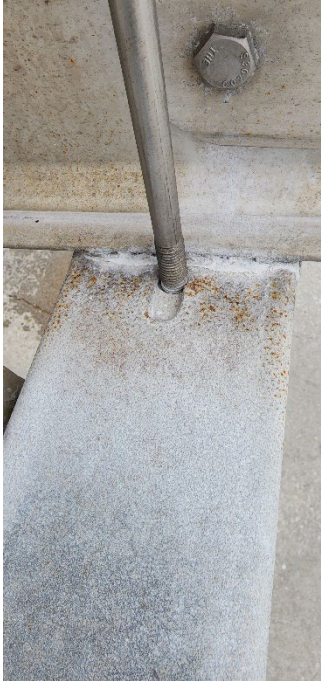
Corrosion around fender brackets
