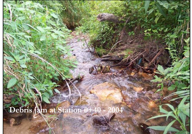
Facing downstream at debris jam at Station 0+40 - 2003
