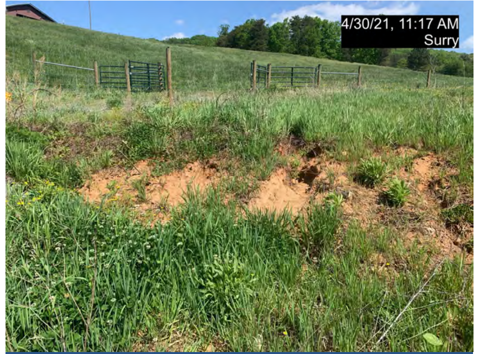
SPA4, R2 Left Floodplain, Minor Erosion (MY-02)
