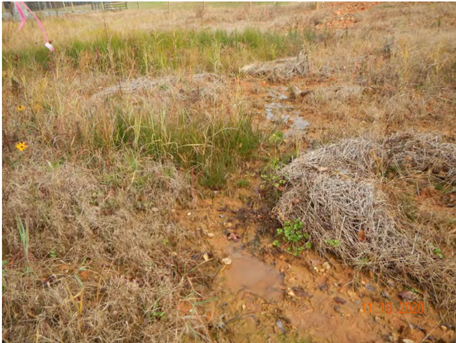
SPA5, R5 Left Floodplain, Minor Erosion (MY-01)
