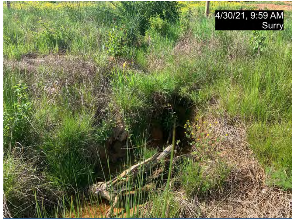
SPA1, R1 Right Floodplain, Minor Slumping (MY-02)
