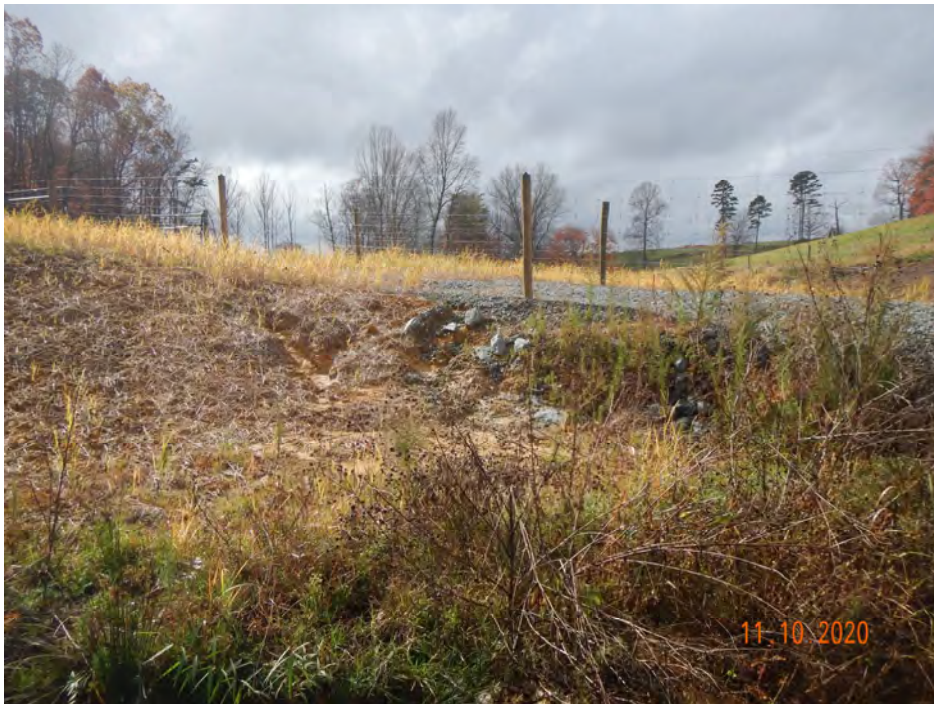
SPA4, R2 Right Floodplain, Minor Erosion (MY-01)
