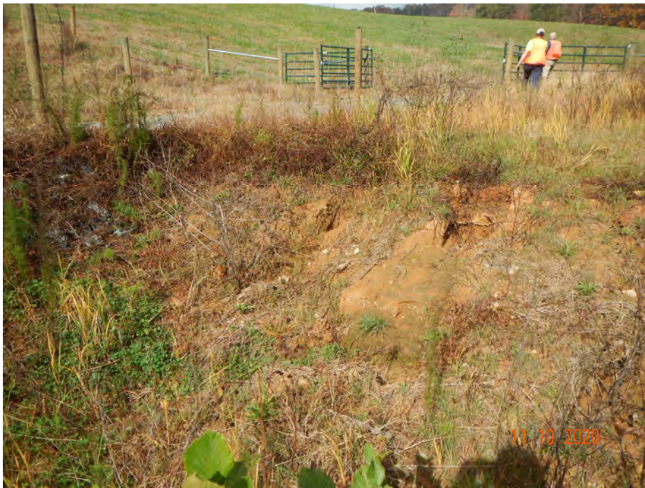
SPA4, R2 Left Floodplain, Minor Erosion (MY-01)
