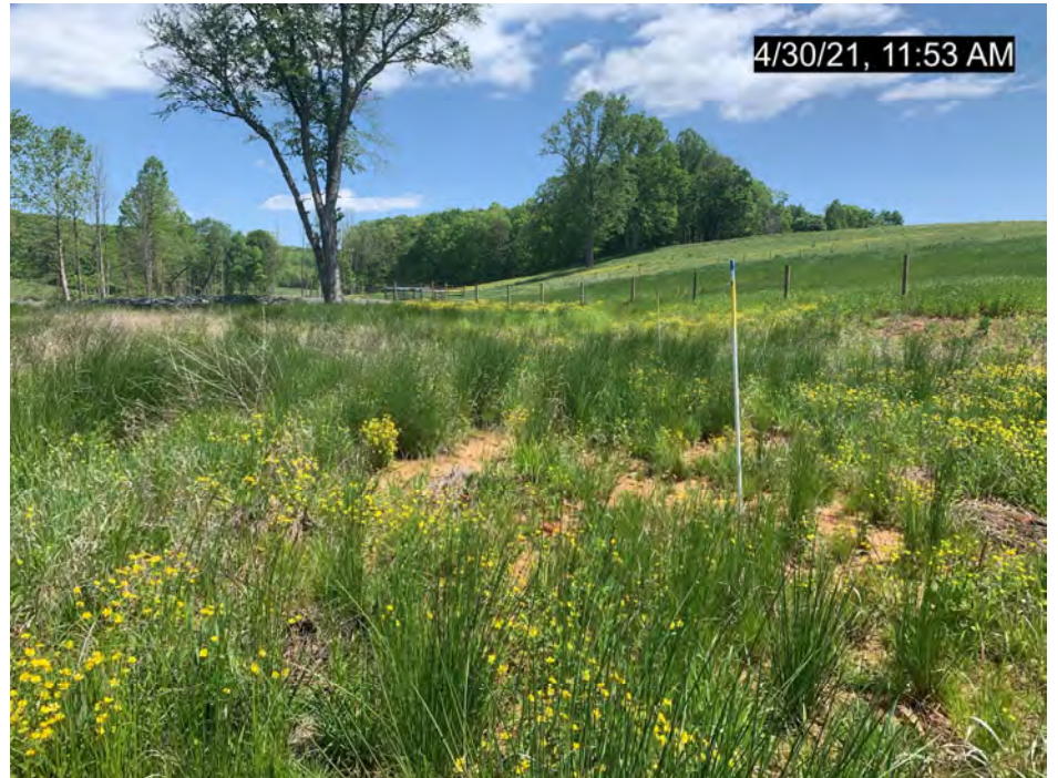
SPA5, R5 Left Floodplain, Minor Erosion (MY-02)
