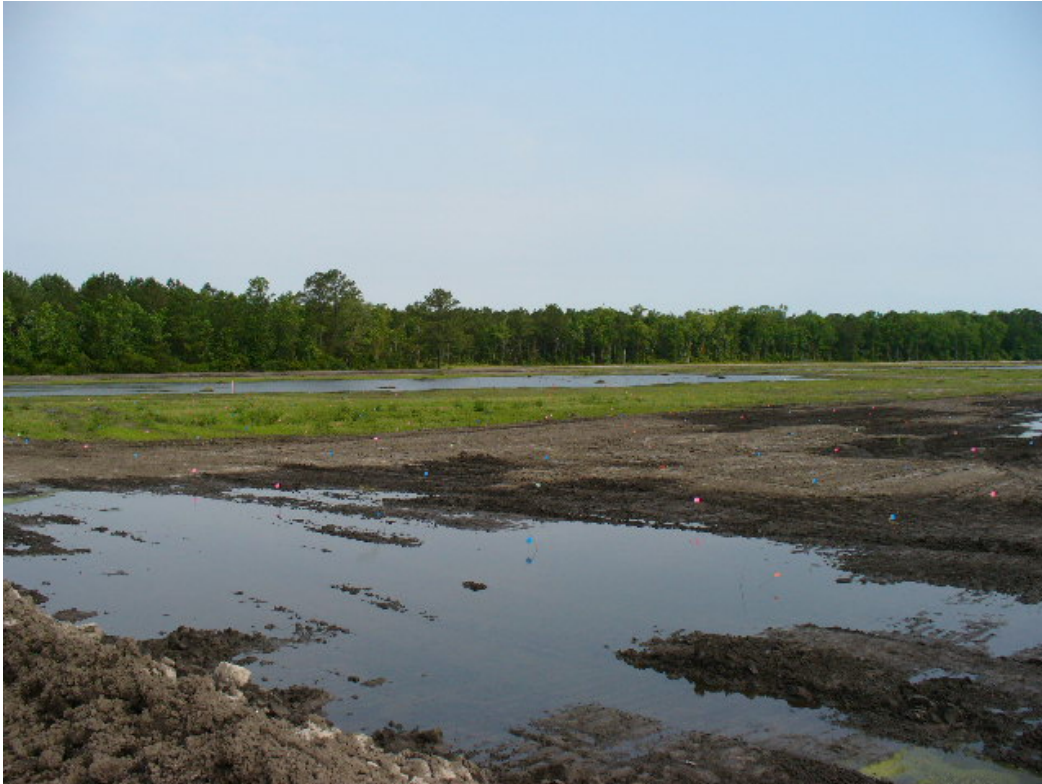
Photo 7. Riverine wetlands (foreground) and non-riverine wetlands just after completion of construction. Pin flags mark locations of woody stock. May, 2007
