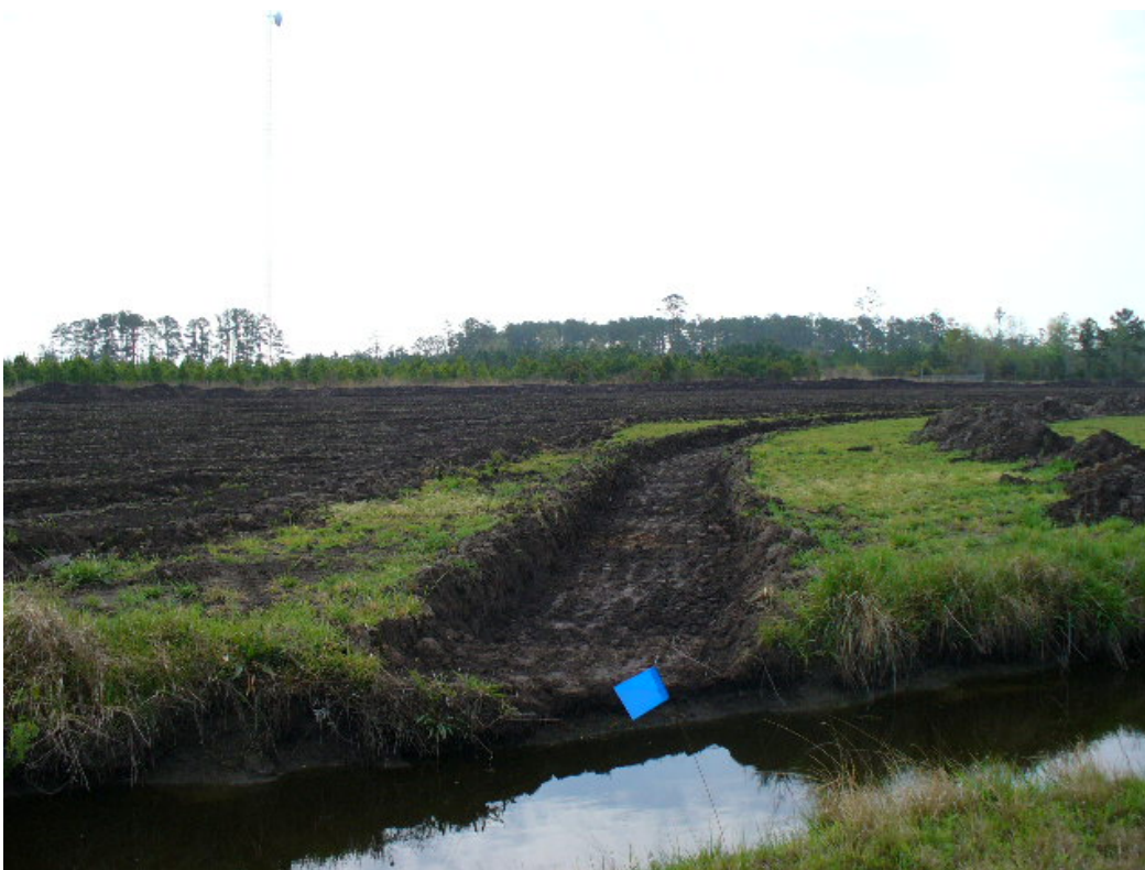
Photo 6. Rough grading of meandering channel shows minimal grading required to restore wetland hydrology to site. April, 2007
