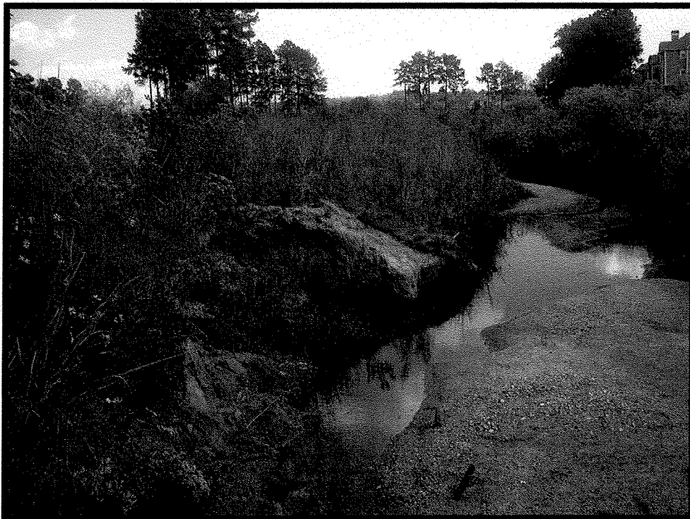
Stream Problem Area 2—Bank Erosion
