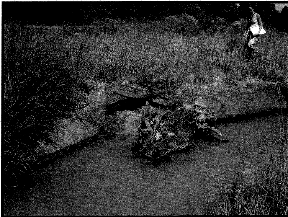
Stream Problem Area 4—Failing Structure
