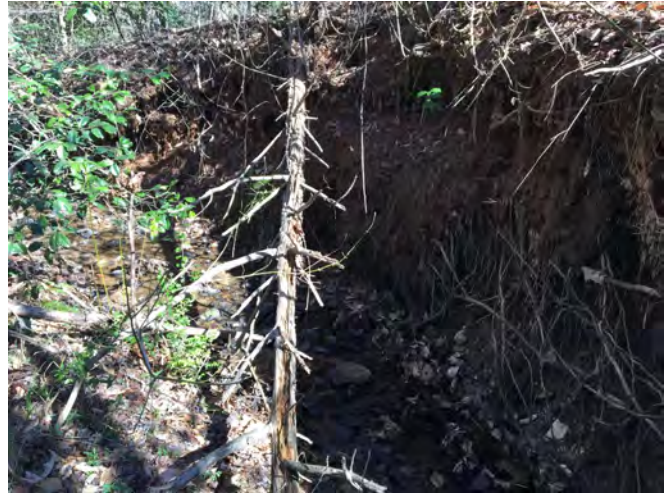
UT 1 – bank erosion and mass wasting.
