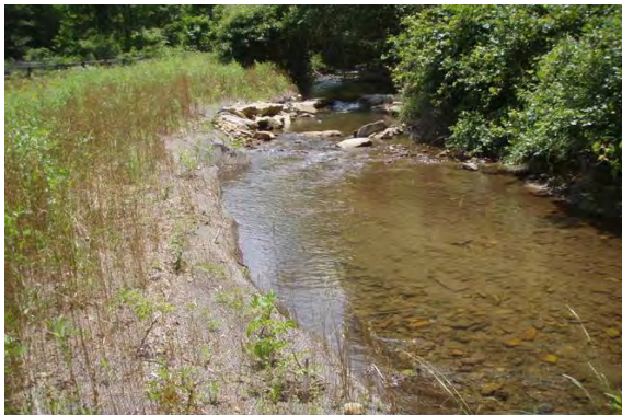
Right channel bank instability after flood, sta. 1+75 to 2+25, facing upstream, 14 June 2012.
