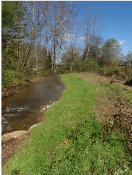
Right channel bank condition after 2015 repairs sta. 1+75 to 2+25 facing upstream, 14 October 2015. No longer considered a problem during MY4 (2015) field surveys.
