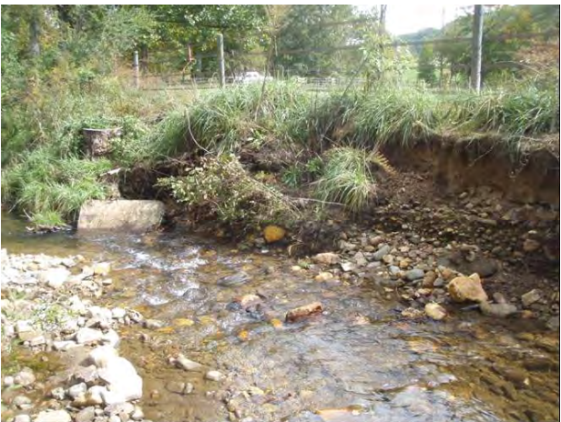
Right bank erosion, sta. 5+50, pre-construction, 30 September 2008.
