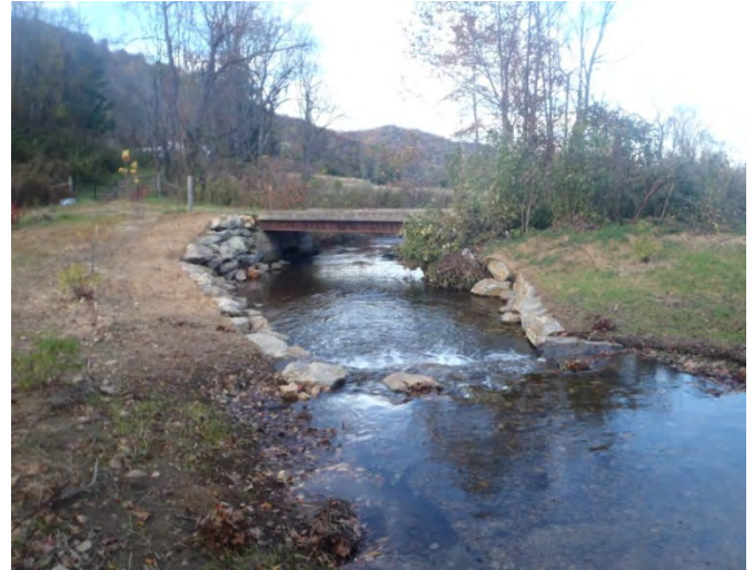
PA-7 station 12+75 facing downstream was repaired and is no longer considered a problem 28 October 2014
