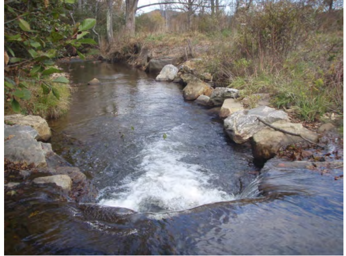
J-hook arm collapse during 5 May 2013 flood event, sta. 5+75, facing downstream, 29 October 2013.
