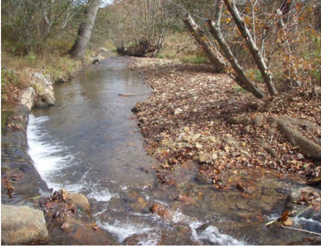
Aggradation below J-hook, sta. 4+00 to 4+50, following 5 May 2013 flood event, facing downstream, 29 October 2013.
