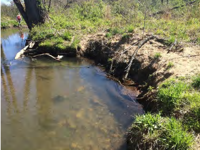
Right bank erosion due to high flow events, sta. 3+45 to 3+70 facing downstream, 18 April 2016.
