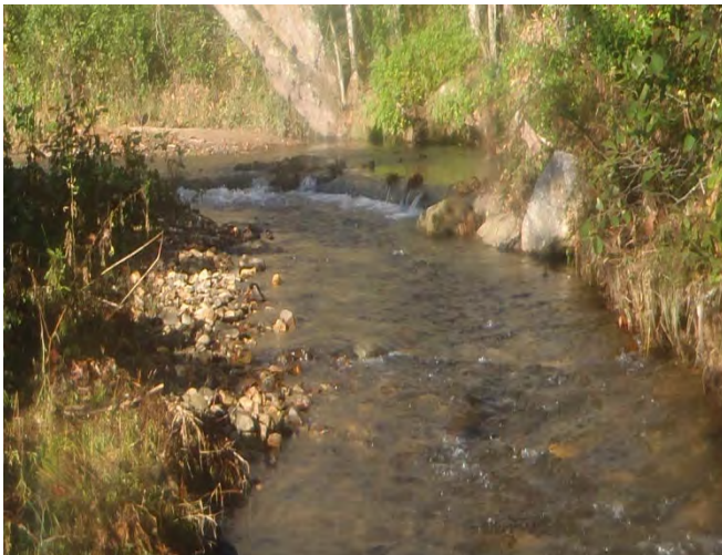
Area below J-hook, sta. 4+00 to 4+50, facing upstream, 15 October 2015. No longer considered a problem during MY4 (2015) field surveys.
