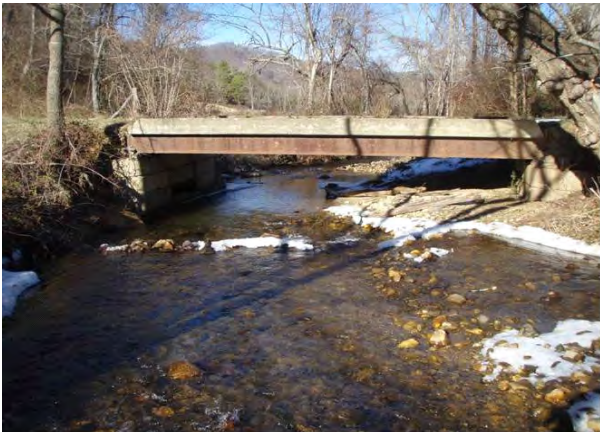
Driveway bridge at lower end of Bura/Roberson properties, sta. 12+50, facing downstream, 22 January 2009.
