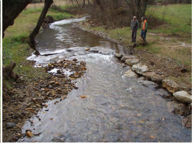
J-hook after 28 Nov 2011 flood event, aggradation in pool below J-hook, 5 December 2011.
