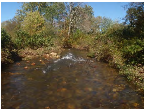
Aggradation and bar formation below J-hook, sta. 9+25 to 9+50, following 5 May 2013 flood event, facing downstream, 14 October 2015.
