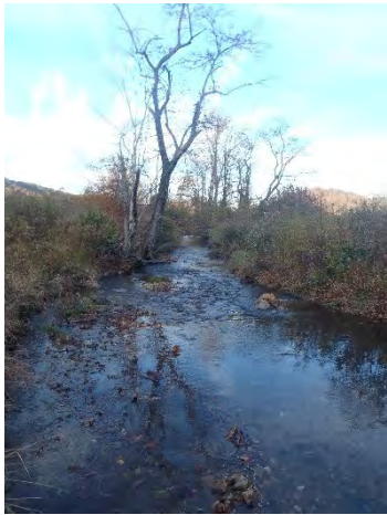
Log vane, root wads, and bank shaping, sta. 2+25 to 3+50, facing downstream, 12 November 2014.
