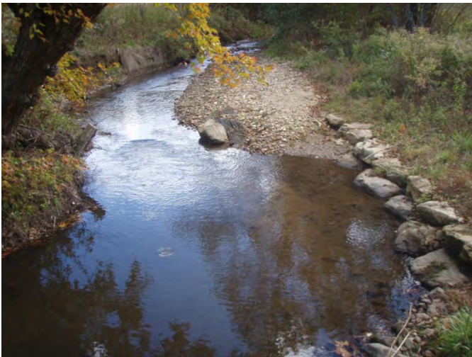
J-hook after 5 May 2013 flood event, aggradation above J-hook and scour pool below, 29 October 2013.
