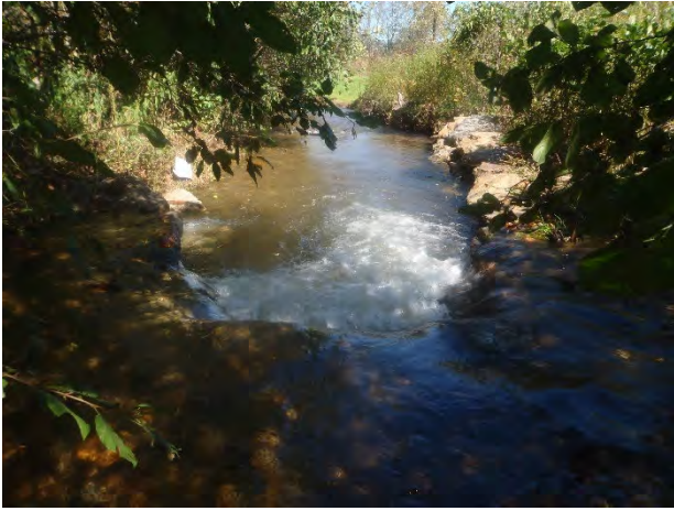
Repaired rock vane, sta 1+50 facing downstream 14 October 2015 No longer considered a problem during MY4 (2015) field surveys.
