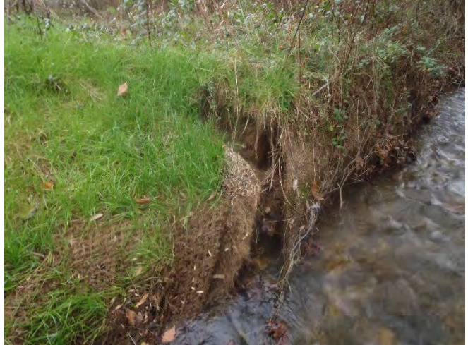
Right bank erosion due to high flow events, sta. 5+05 to 6+10 facing upstream, 17 November 2015
