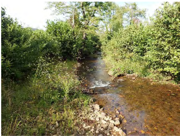
Log vane, root wads, and bank shaping, sta. 2+25 to 3+50, facing downstream, 15 Sept 2016.
