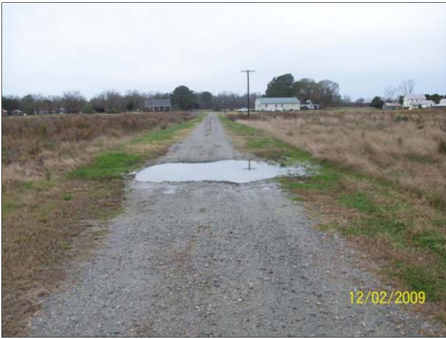
Photo Point 4 – 12/2/09 - MY 02 – Road Crossing Type A – Station 17+75 – Facing west toward Macedonia Road.
