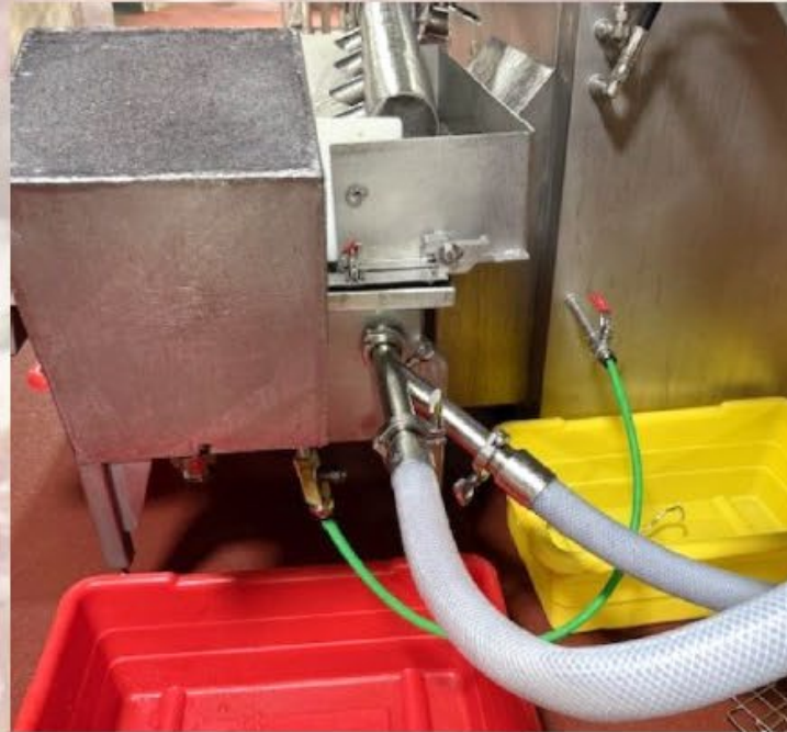
brine recovery hoses
