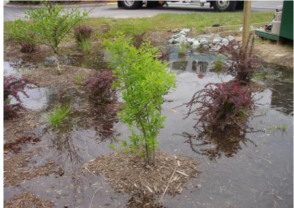
A bio-retention area effectively captures runoff, preventing large volumes of polluted runoff from entering a stream.
