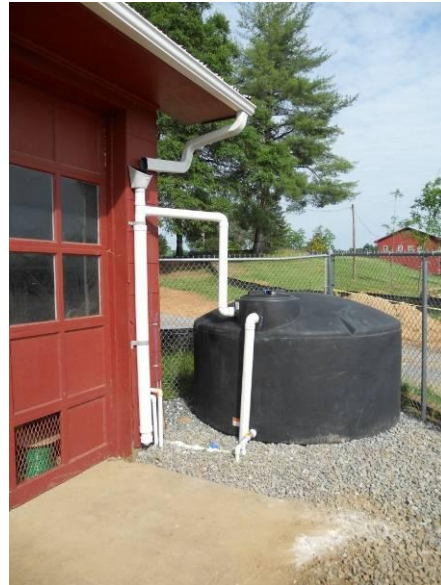
An above ground cistern located at the City of Morganton Parks and Recreation maintenance building catches runoff from the roof. The water is used to clean equipment.
