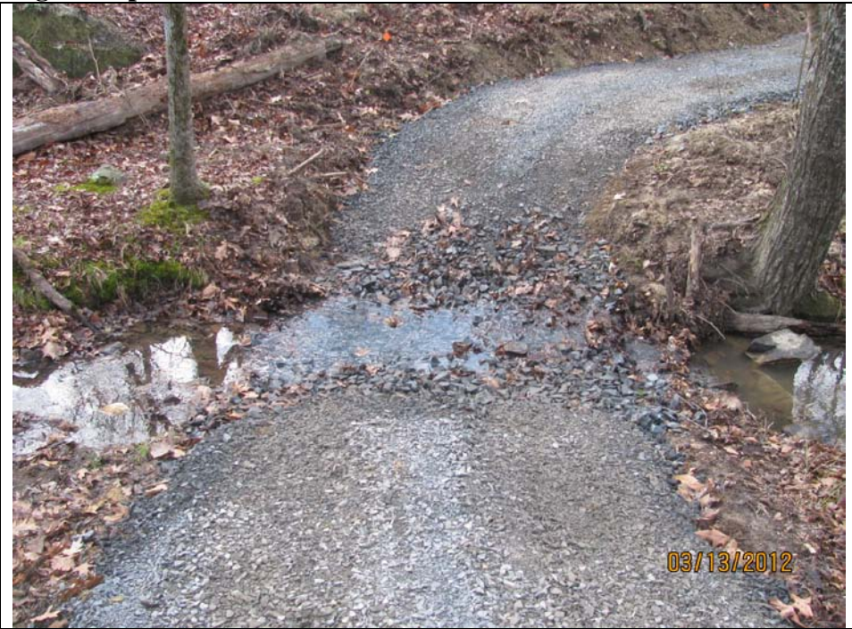
Photo 2: NOT IDEAL: - Hardened stream crossing with gravel in stream bed that is impeding stream flow and creating check-dam effect.
