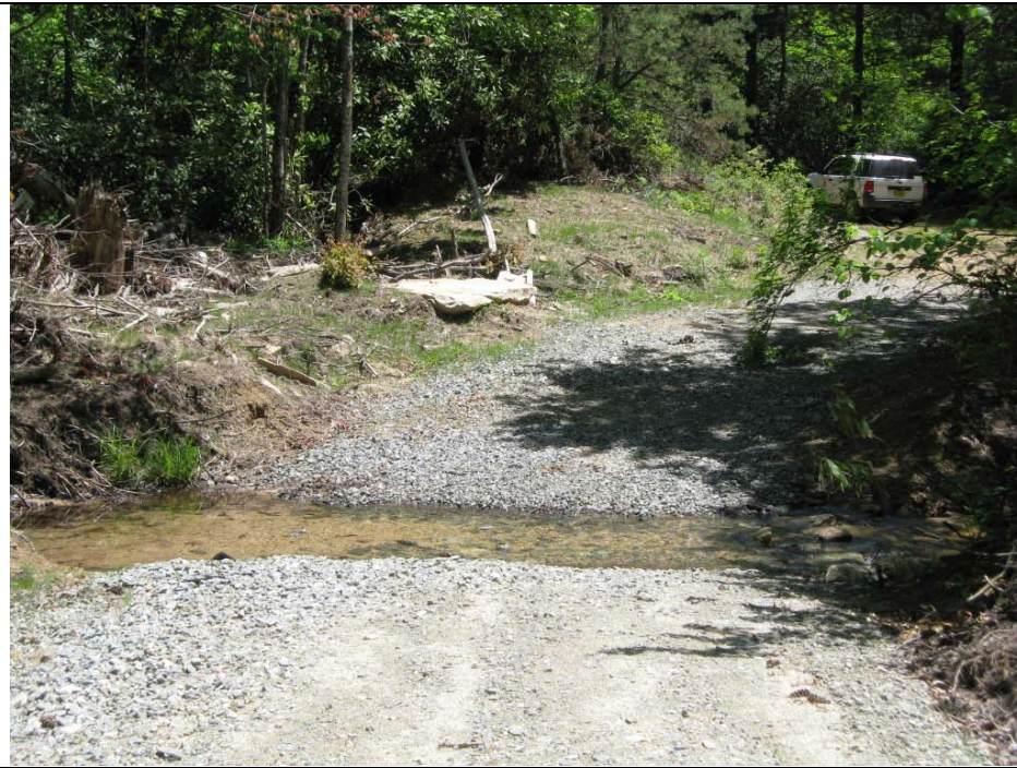
Photo 1: IDEAL - Hardened crossing in low gradient stream with natural substrate allowing for un-impeded stream flow.
