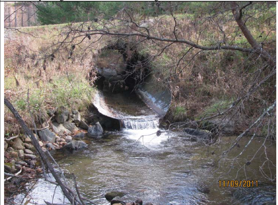
Photo 4: NOT IDEAL – Culvert perched above stream bed and impeding aquatic passage upstream. Large scour pool indicates culvert undersized.
