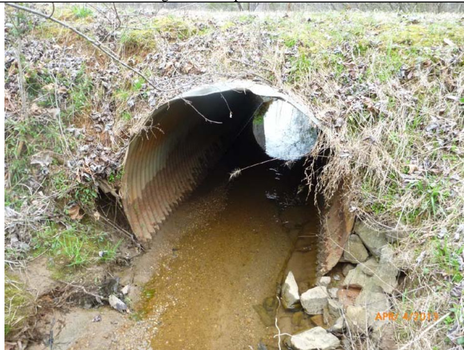
Photo 3: IDEAL – Culvert buried below stream bed with natural substrate; stable earthen material around culvert with minimal erosion.
