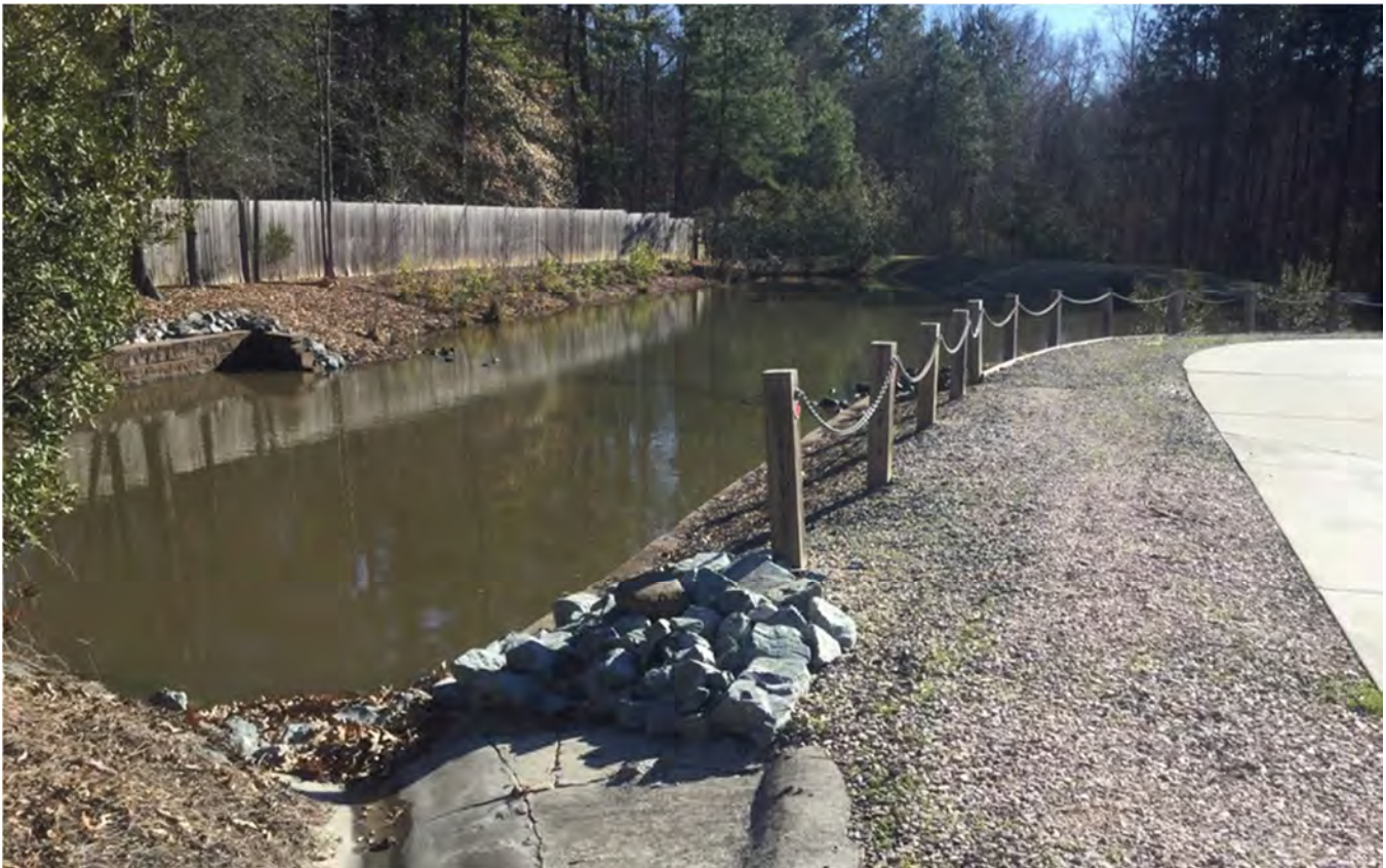
Figure 4-1. Example of retrofit opportunity at a wet pond (SCM Site 00316 located along SW Durham Drive in the Lower New Hope Creek watershed). The temporary storage volume of this wet pond is relatively small and could be increased. The proposed retrofit at this location, a wet pond with increased storage, would involve lowering the water level to gain storage.
