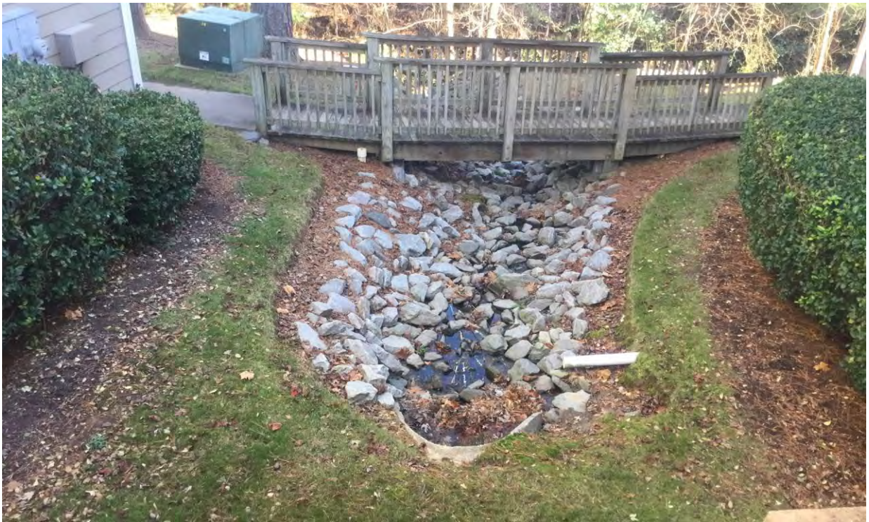
Figure 4-3. Potential new SCM site in which a regenerative stormwater conveyance was recommended (SCM Site NHCSC0040 located along McQueen Dr. in the Sandy Creek watershed).
